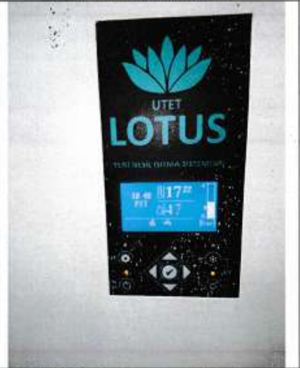
Pic6- Daily-hot water feeding test
