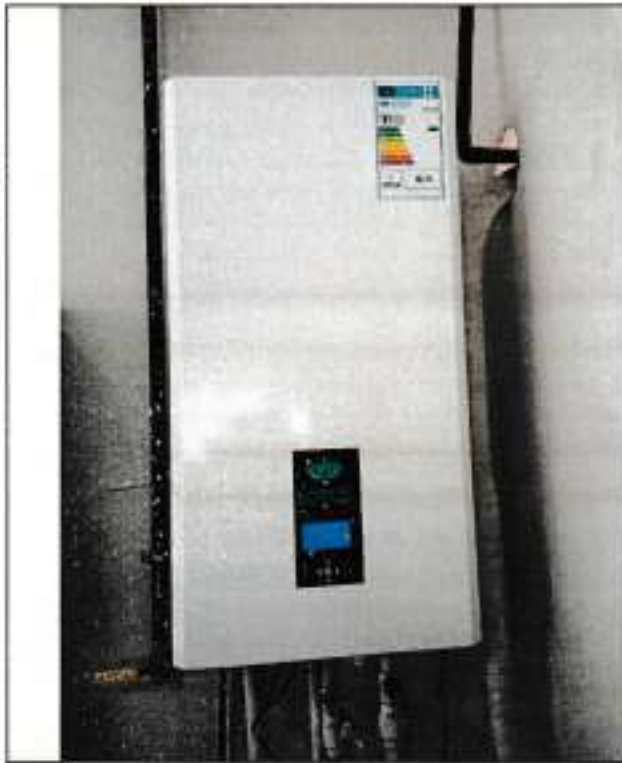
Pic.1 - General view of the E300 boiler.
